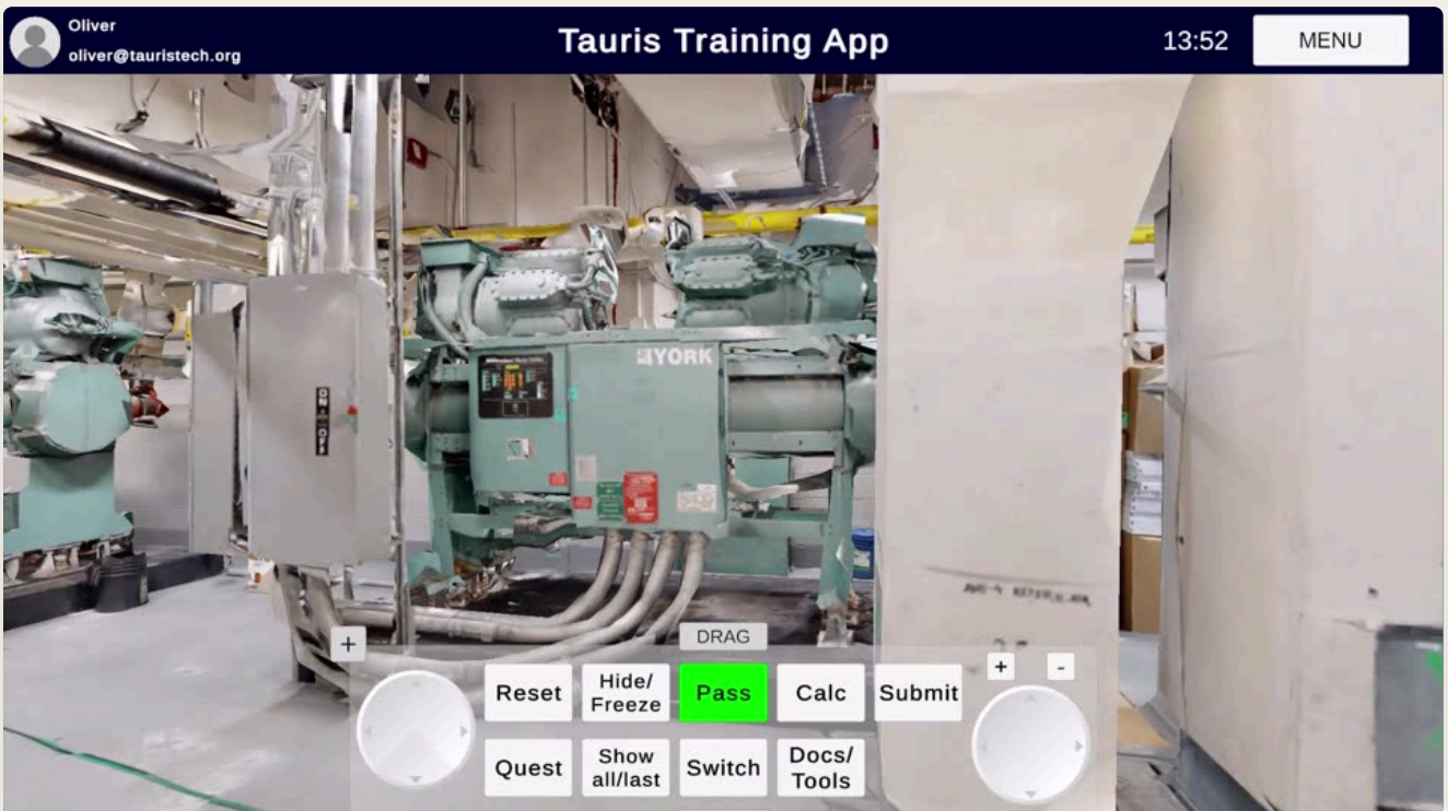
FIG. 04.1 Reciprocating chiller – simulator wide view
